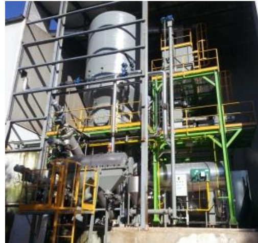
MBM Gasification 16 MWth. Oporto, Portugal
