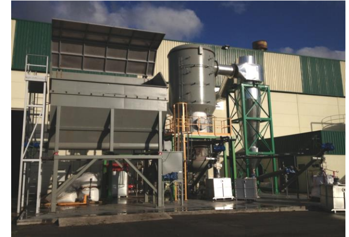
MBM Gasification 10 MWth. Salamanca, Spain
