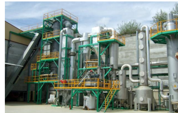
Woodchips Gasification Power Generation. 1.6 MWe. Xátiva, Spain
